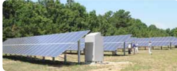
92kW Ground-mounted Photovoltaic Installation at the Calverton National Cemetery on Long Island
