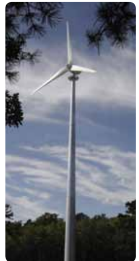
The 50 kilowatt Endurance turbine at the Bourne National Cemetery
